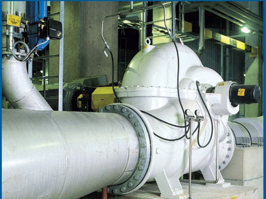
Horizontally-split double-suction fan pump in paper mill
