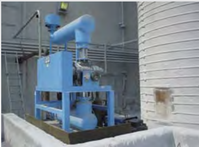
Blower package conveying hydrated lime.
