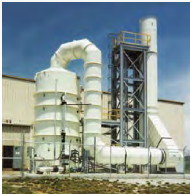
Packed fume scrubber system in a plating facility.
