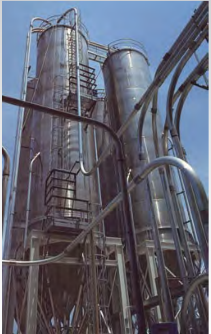
Petro-chemical powder transfer and storage system.
